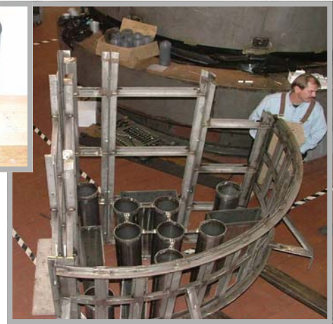
Shielding Structure & CEA Shields
